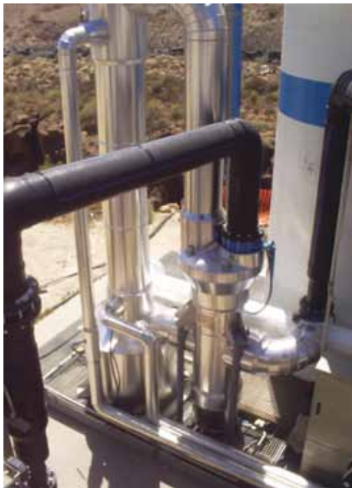
Figure 2: View of scrubber-economizer. Images courtesy of Energy & Waste SLNE.
